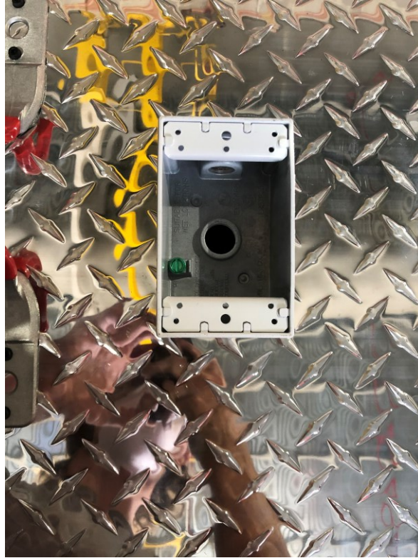
Figure B.4 The external switch box mounted with the 1/2” rigid comp connector
