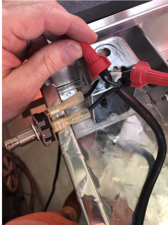
Figure B.19 The wiring of the 2' length of power cable and the power strip to the 15A contact switch
