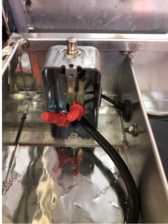
Figure B.20 The wired 15A contact switch mounted into the RACO internal switch box
